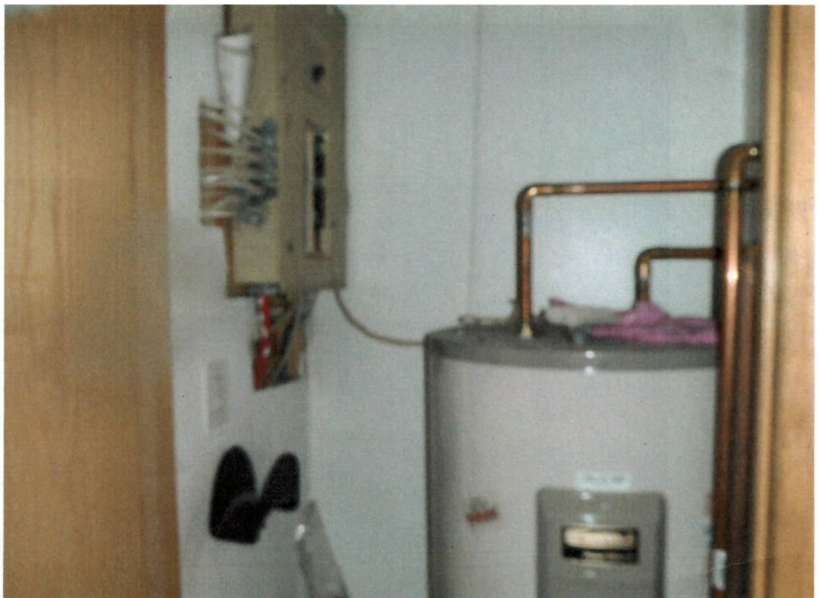
Panel box / hot water tank
